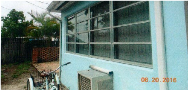
Before: Wall Unit Air Conditioner
