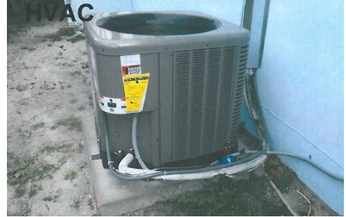
After: Central Air Conditioning
