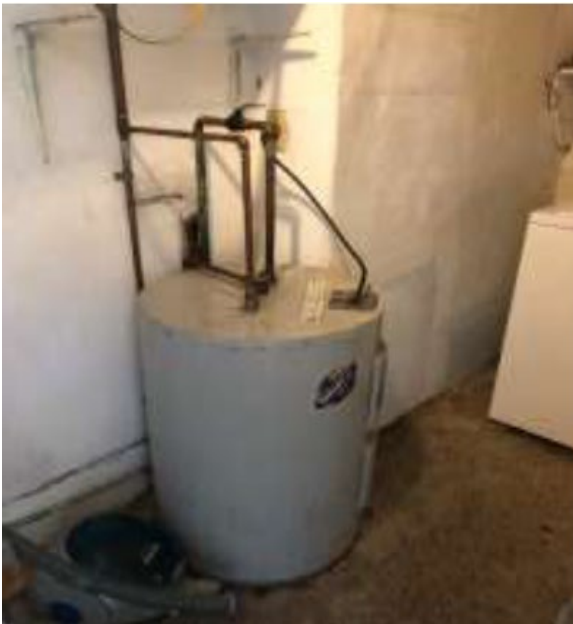
Before: Hot Water Heater
