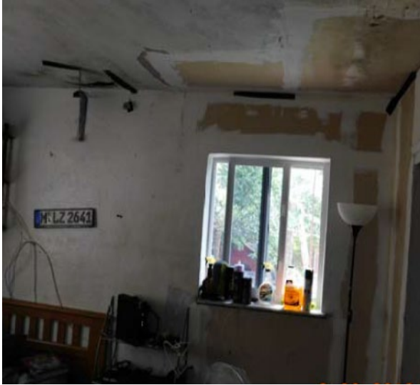
Before: Damaged Drywall/Mold
